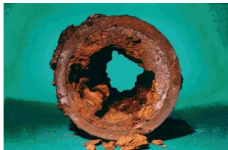
Corroded metal piping
