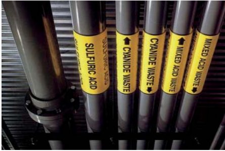
CPVC chemical waste piping systems
